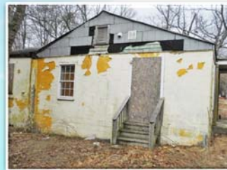
Exterior walls with peeling flaking paint
