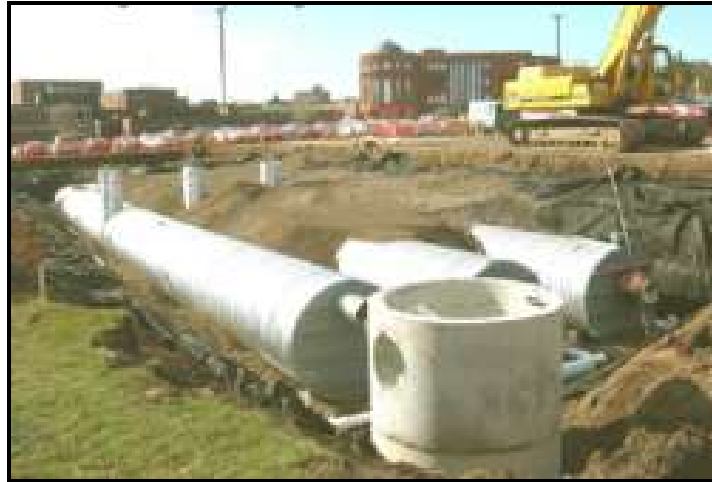
Figure 24 Underground Storage (Source: Lake Superior Duluth Streams--Stormwater)
